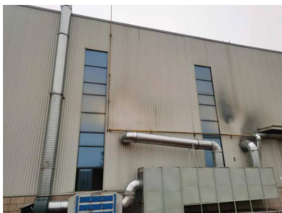
喷淋+活性炭吸附+排气筒
